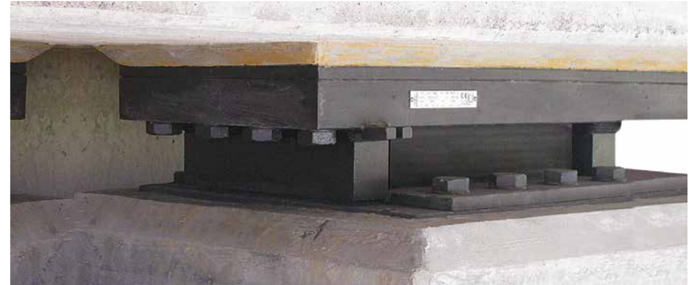
Guided elastomeric bearing, Type S-RBU, installed
