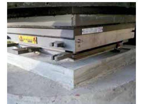
Pot bearings after installation
