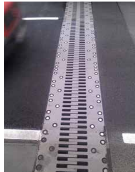
Finger-type expansion joint in operation
